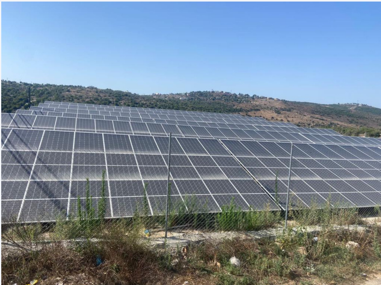
Photovoltaic solar panels previously installed by our ground partners.
